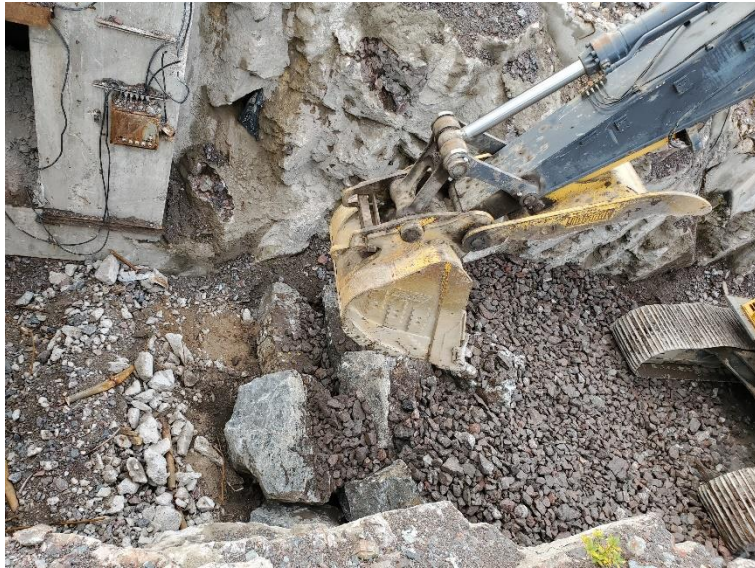
Photo 12: Placement of coarse waste rock over the boulders at Raise 3 to safely access Raise 2.
