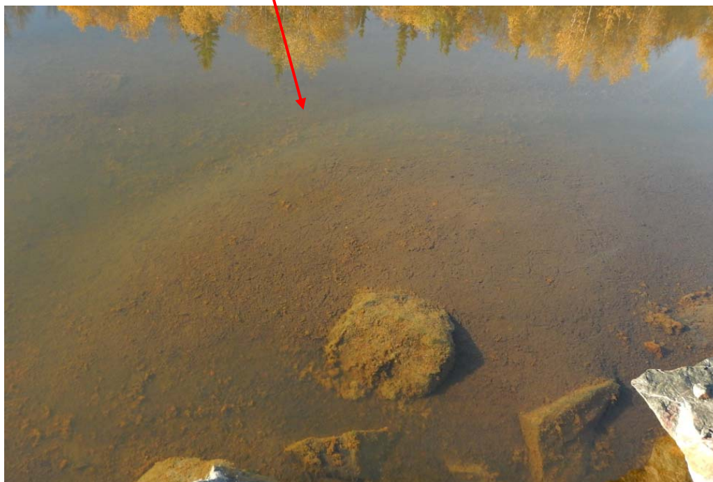
Photo 9: Looking South at Channel Base Sedimentation (Station 0+215)
