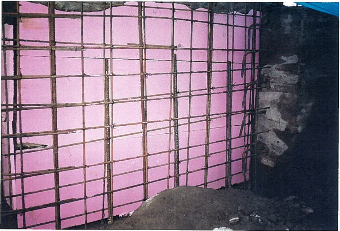
Photograph 3: Form break and rebar on the walls. Note: the rebar detail was revised to tie into existing wall.
