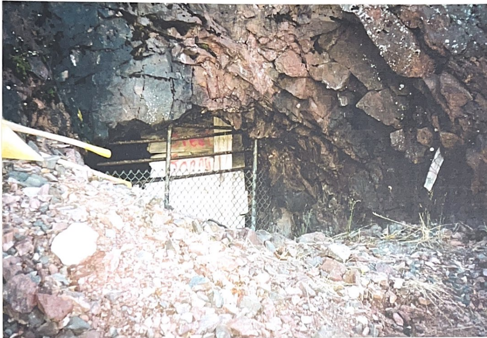
Photograph 1: View of the initial fencing that was removed and replaced with bolted and welded structure.
