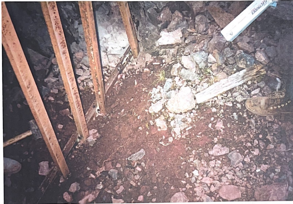
Photograph 3: Debris removed approximately 2 ft. to rock and backfilled on completion at bottom end.
