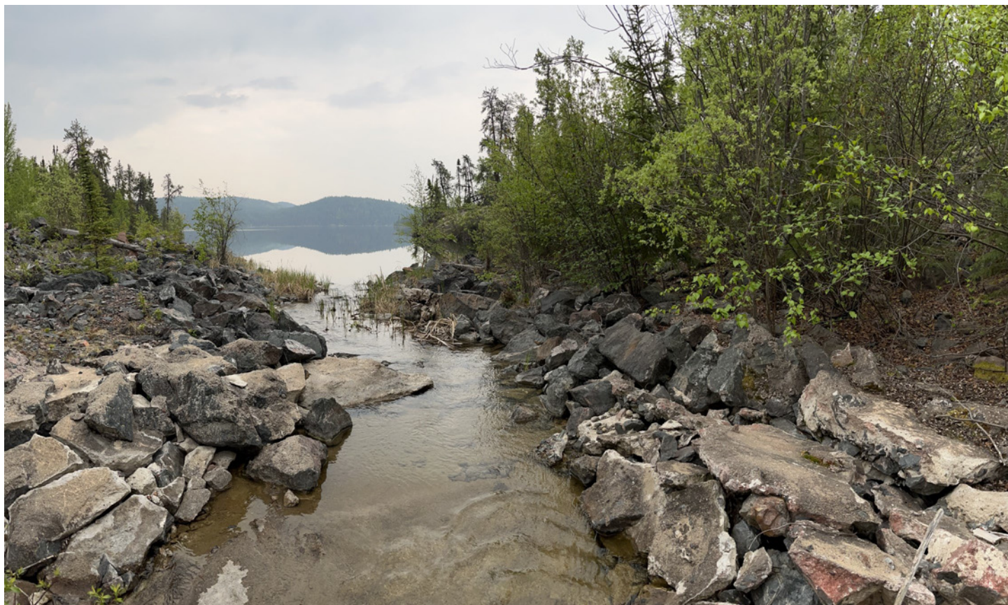
Photo B5 – Fookes Reservoir Spillway showing broken rip-rap on north and south sides of channel. Note debris has been removed since 2022 inspection.
