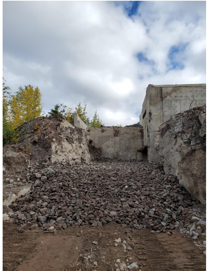
Photo 17: Additional placement of coarse waste rock over Raise 3 and 2, up to the entrance at Raise 1.
