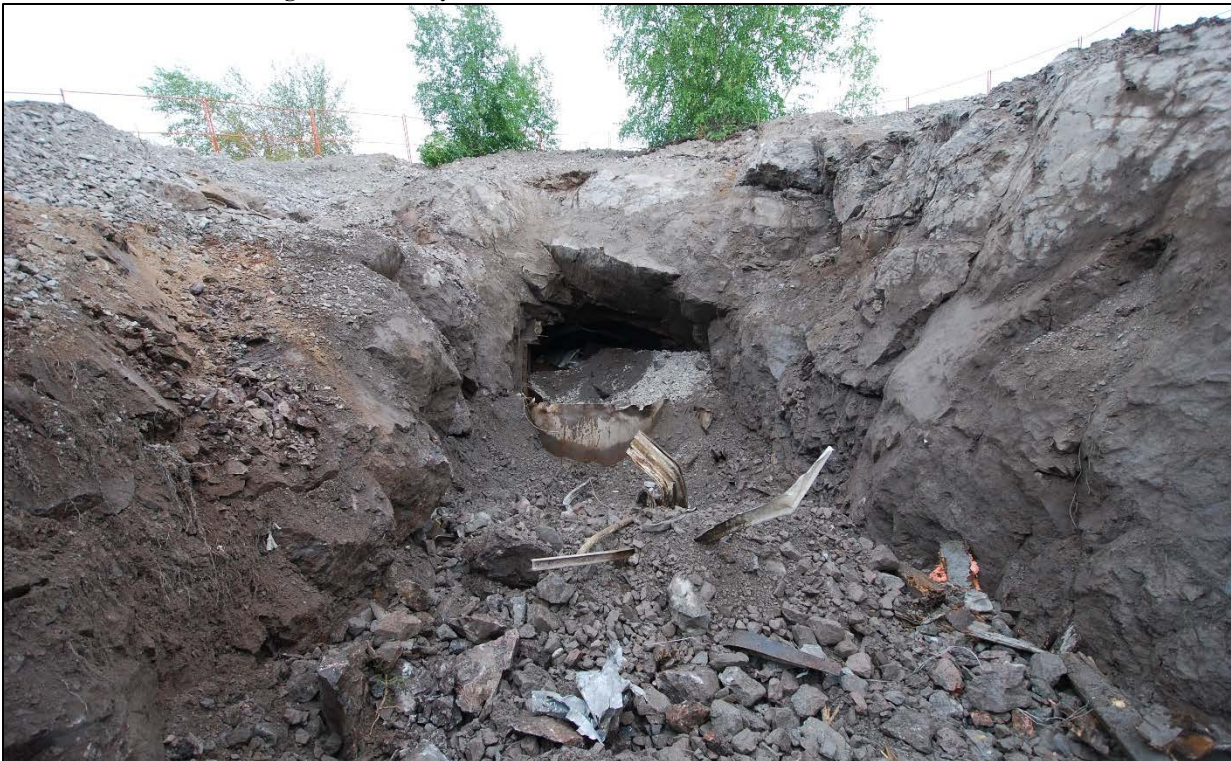
Figure 2: Partially Excavated Adit with Steel Encountered in Backfill
