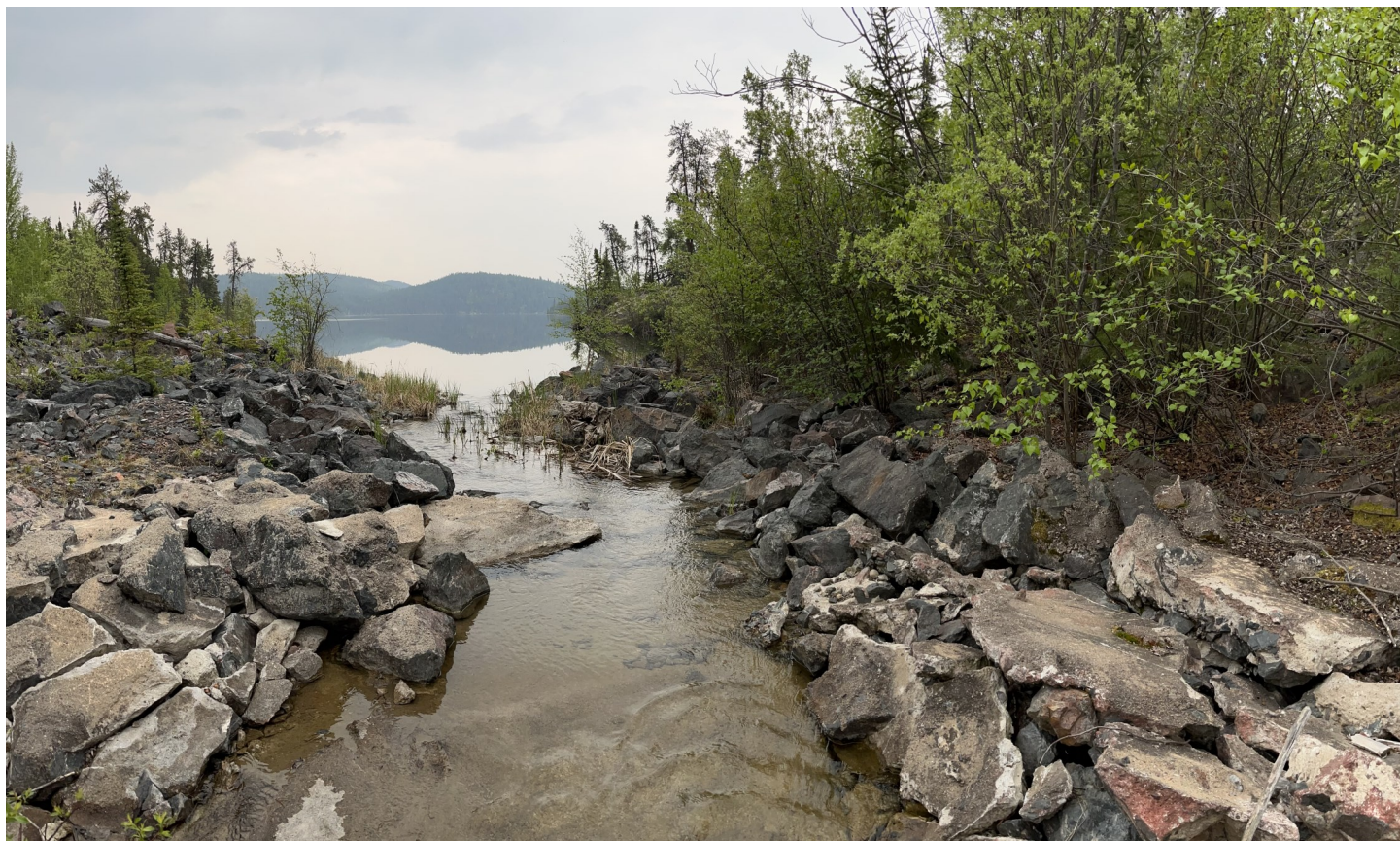
Photo B5 – Fookes Reservoir Spillway showing broken rip-rap on north and south sides of channel. Note debris has been removed since 2022 inspection.
