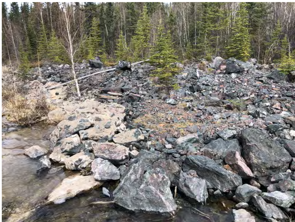
Photo B5 – Fookes Reservoir Spillway broken rip-rap on north side of channel
