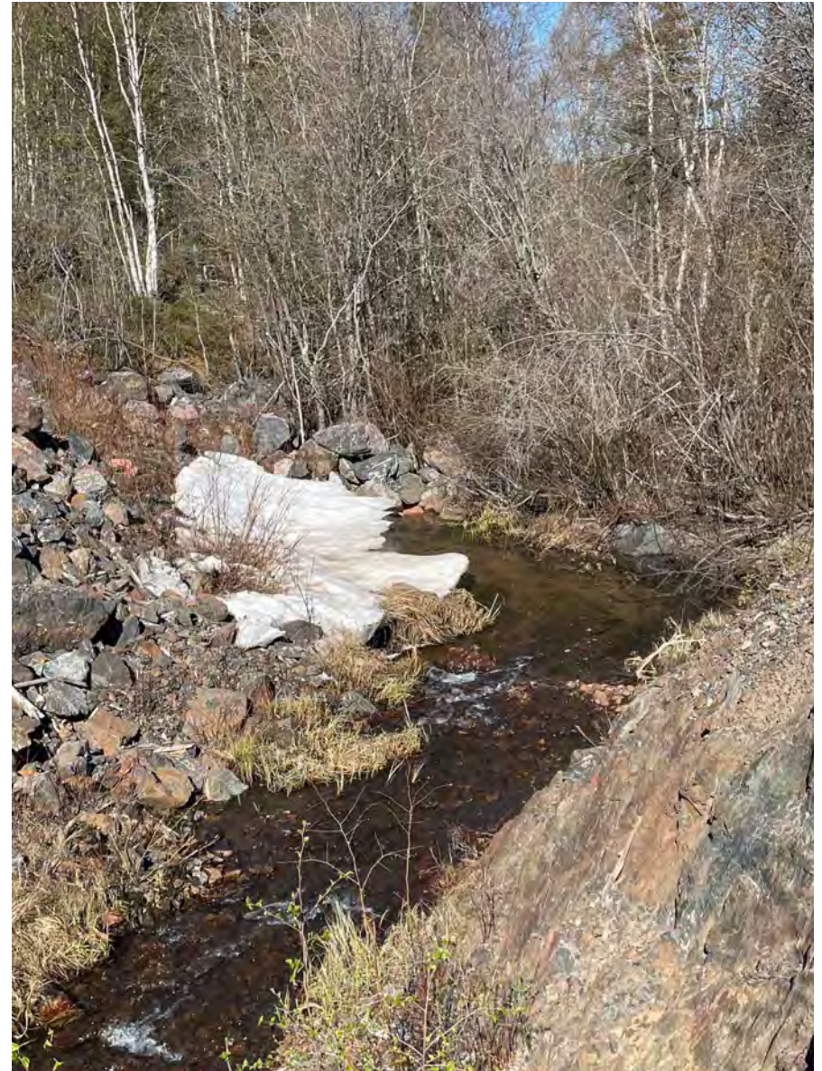
Photo E04—View near stilling basin, looking downstream at stilling basin (May 31, 2022) Note the glaciation remaining from the late spring
