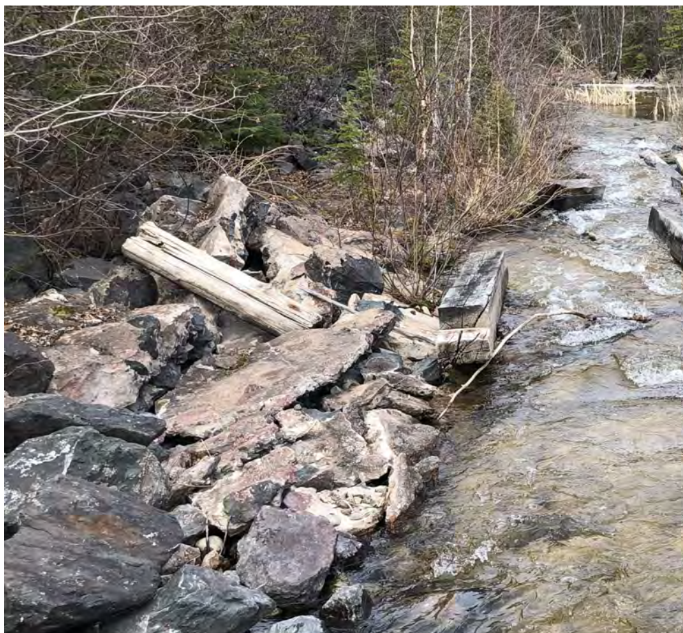
Photo B6 – Fookes Reservoir Spillway broken rip-rap on south side of channel
