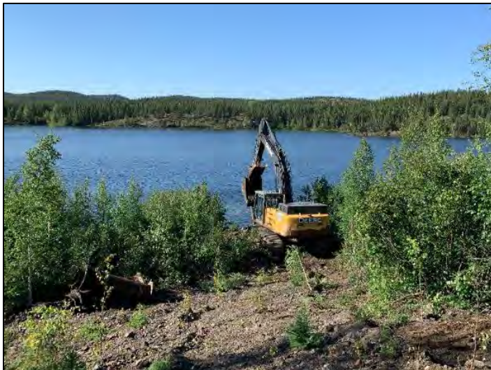
Photo 12. Excavation of backshore portion of the pumphouse (underground water pipes on left of photo)
