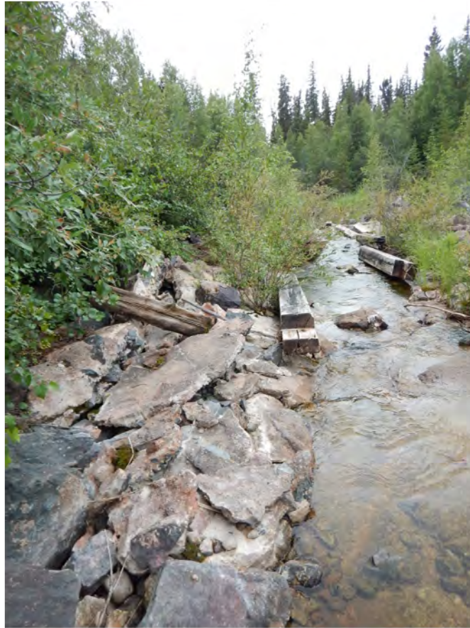
Photo B5 – Fookes Reservoir Spillway broken rip-rap on south side of channel
