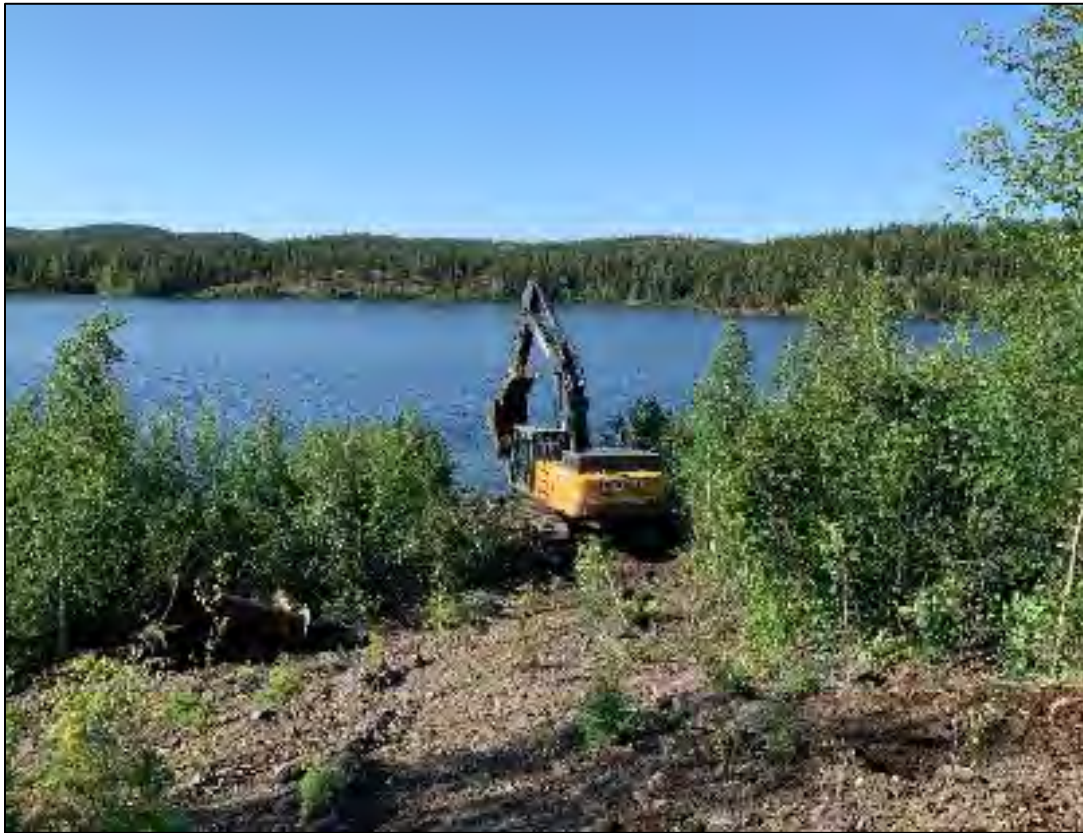
Near the start of the excavation of pumphouse materials on Verna Lake. Old pipe is on the left of the photo.
