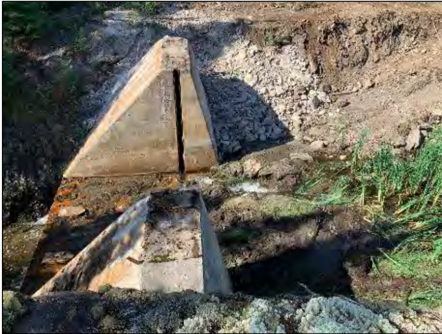
Photo 4. View from right bank (when facing upstream) after metal frame and stop logs were removed; note new flow path of water moving across the remaining structure (flow is from right to left)
