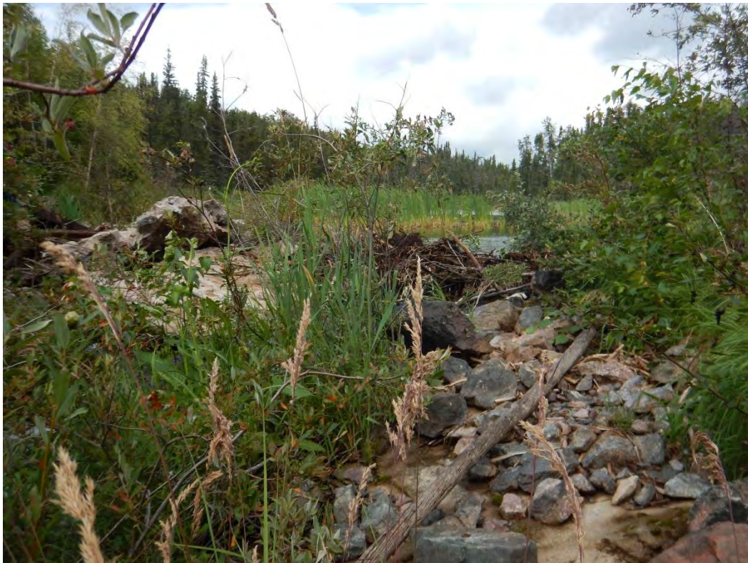
Photo A4 – Displaced grout intruded rip rap at the entrance to the spillway (far left of photo)
