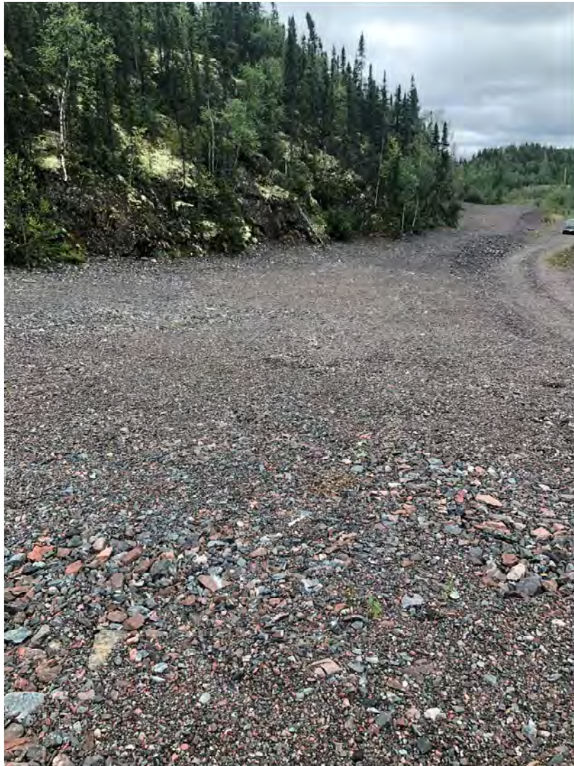
Photo D1 - View of the cover placed over Ace 201 Stope
