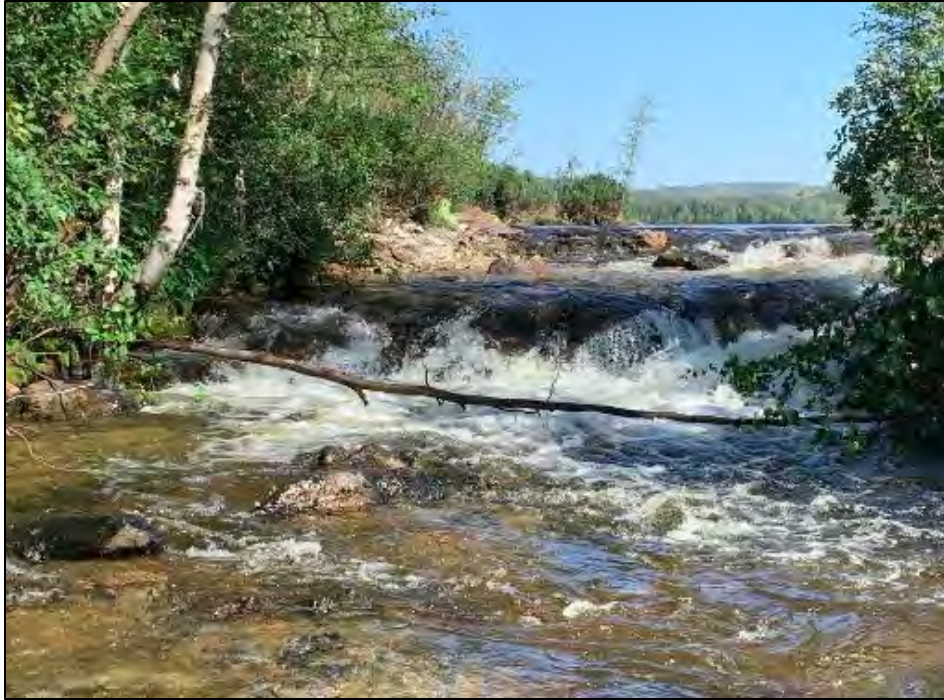
View looking upstream at completed work on Ace Creek. Rock in center channel is where the old weir was located. The small drop at the bottom of the photo is the existing bedrock drop that was below the weir.
