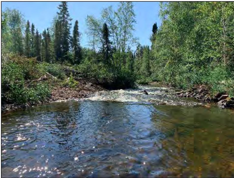
View looking downstream towards location of the former weir on Ace Creek. All work was completed from the south side of the creek (left side of photo). Slash has been placed on the slope where the machine worked.
