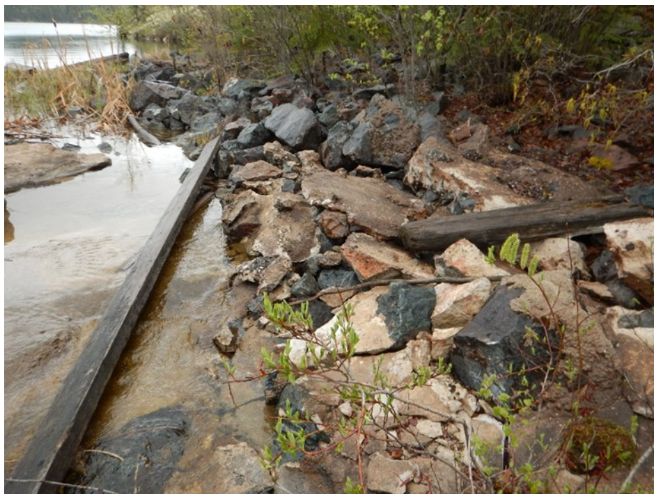
Photo B5 – Fookes Reservoir Spillway broken rip-rap on south side of channel
