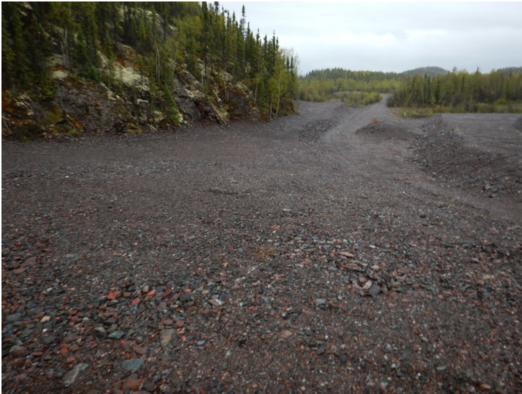
Photo D1 - View of the cover placed over Ace 201 Stope
